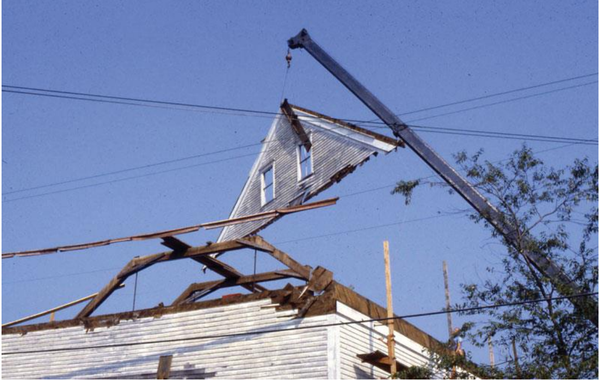
It took more than a year to document and disassemble the barn, which was taken apart piecemeal. Here, the roof peak is removed, window frames still intact.
