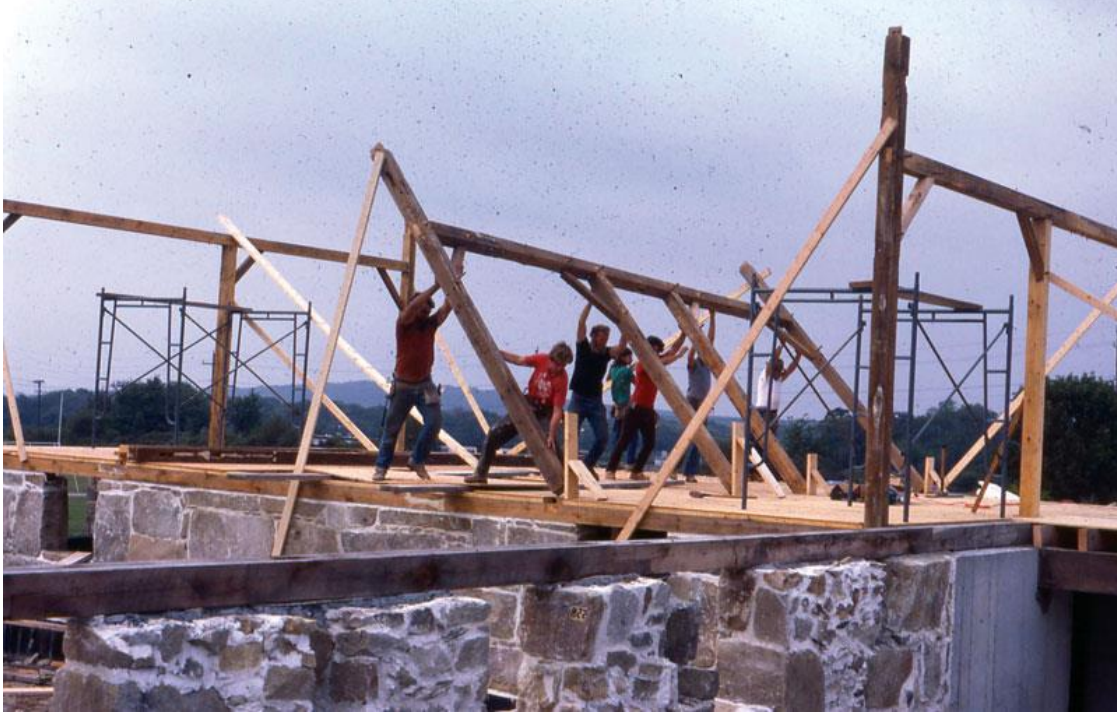
Students push up the two-story post frame – a process called “timber raising” – as they begin to reassemble the Barn. New material was used to brace the historic materials, which constitute the majority of the structure.
