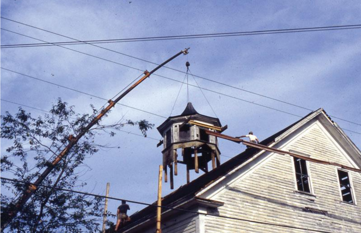
The cupola was stabilized, and a crane brought in to remove it fully intact, to avoid damaging the structure.
